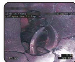
•• Collapse Due to Tap-In.
