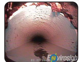
•• Dropped 10' Section of PVC and Eroding Joint.
