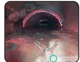
•• 8" Terra Cotta Mainline with Offset and Infow.
